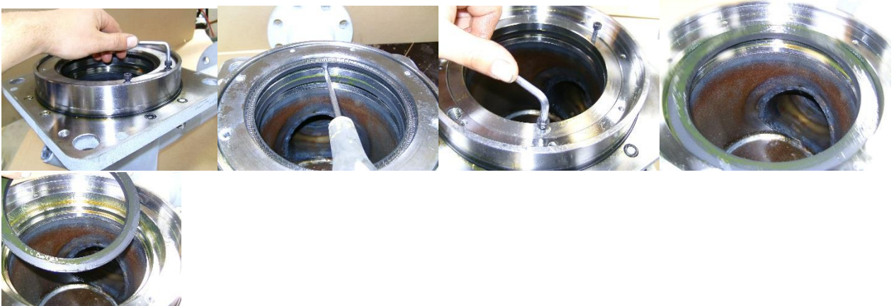
The ring pos 4.25 is removed so the seals can be replaced. Seals and intermediate ring pos 4.24 is replaced
