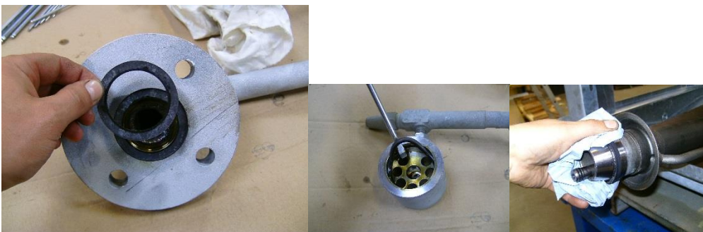
Seal pos 4.21 and O-ring pos 4.36 is replaced, Liquid pipe and oil pipe is cleaned
